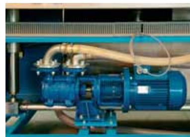
Water suction pump
